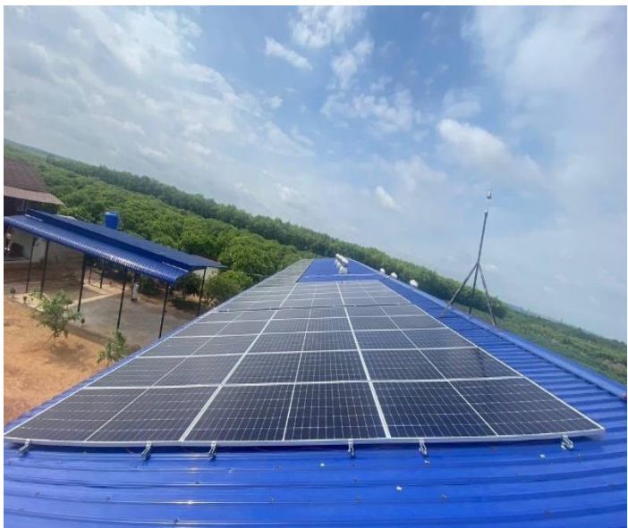
Figure 3 " Credit Photo: Solar system installed at HCST "
